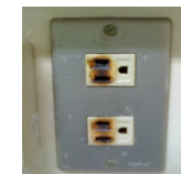
▲Burned outside of outlet
